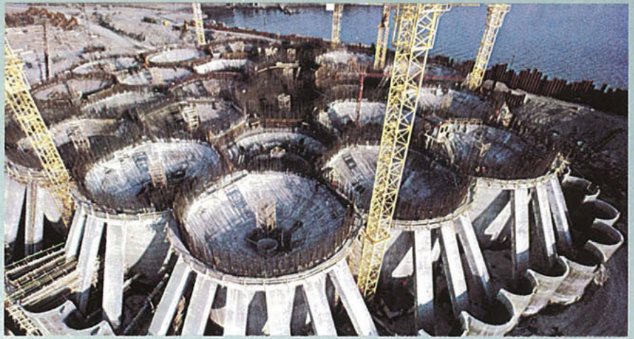
The concrete structure of the Statfjord B platform, under construction at Hinnavågen, Stavanger, in March of 1979. The Statfjord B platform will be the world's largest oil production platform. It covers a surface area of 18 000 square meters, or the equivalent of 4.446 acres.
