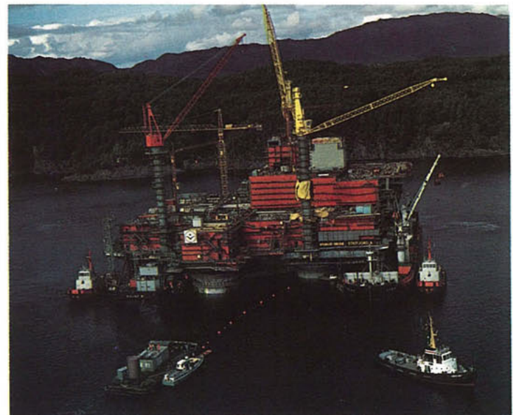
3) September 1976: The steel deck and the concrete structure were mated at Stord Verft.
