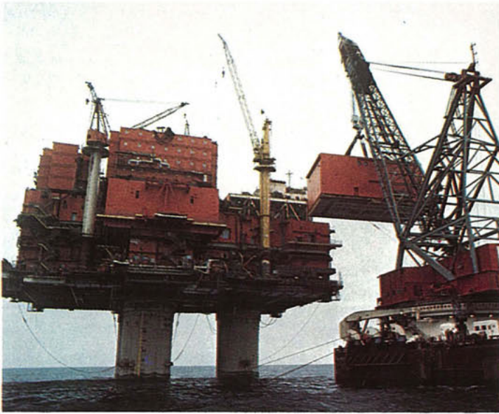
5) September 1977: Construction work continued on the field. Modules are lifted into place by Seatroll .
