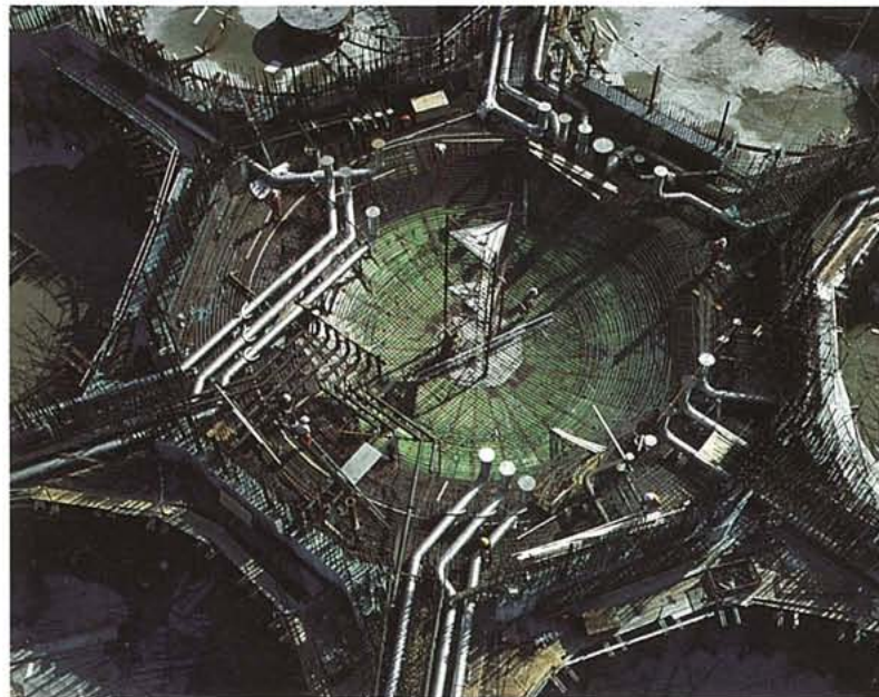
As the first platform in the world Gullfaks A will have stainless steel pipes — an economical investment. The concrete gravity base structure is being built by Norwegian Contractors in Stavanger.
