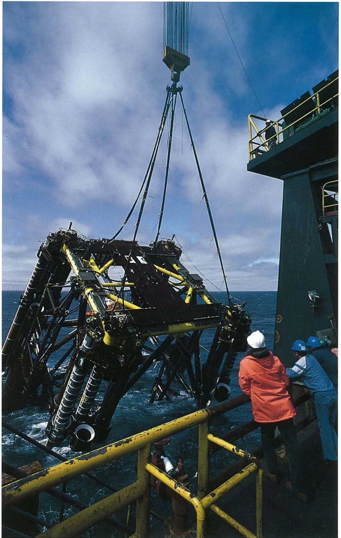
The steel jacket for Statpipe's riser platform 2/4 R is being positioned, not far from the Ekofisk tank.
