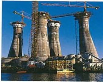
The Sleipner A concrete gravity base structure. The shafts are 47 metres tall.
