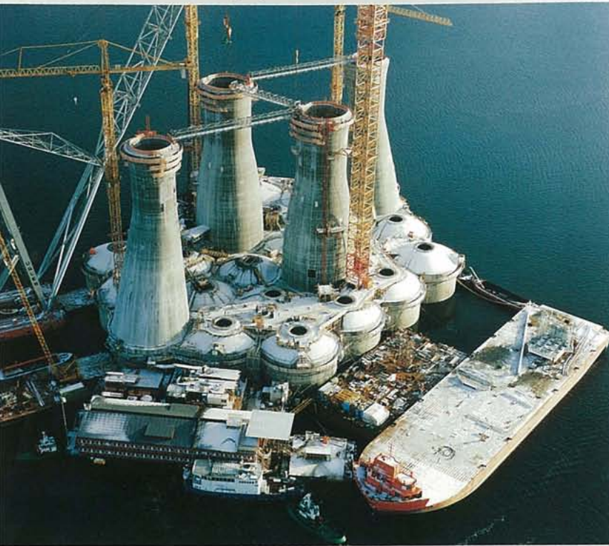
The new concrete gravity base structure for Sleipner A under construction outside Stavanger.
