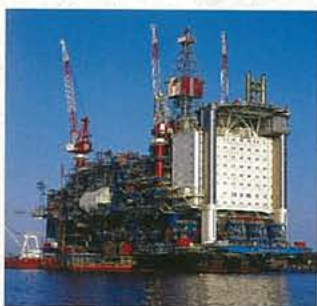
The Sleipner A topsides waiting to be mated with the concrete gravity base structure and completed prior to being towed out to the field.
