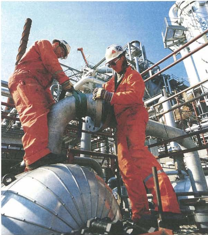
METHANOL PLANT: The new methanol plant at Tjeldbergodden in mid-Norway is approaching completion.
