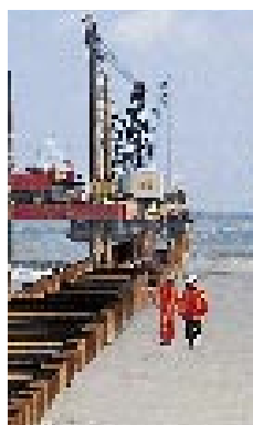
THE NORFRA LANDFALL AT DUNKERQUE IN FRANCE.
