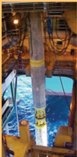
From drill floor on Erik Raude, operating off Canada. (Picture: Ocean Rig)
