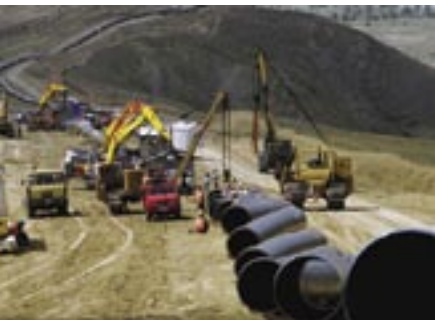
Statoil is involved in the construction of the large export pipeline for crude oil from Baku in the Caspian to Ceyhan in the Mediterranean. The BTC pipeline will be able to transport more than one billion barrels of crude oil daily to world markets and will be operational in 2005. (Photo: Statoil)
