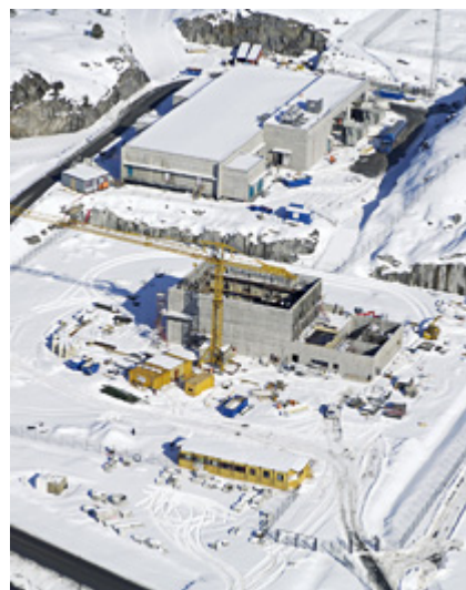
Statnett's work with the new power line from Viklandet till Nyhamna (picture) will be done in 2006. (Foto Hydro: Leren)
