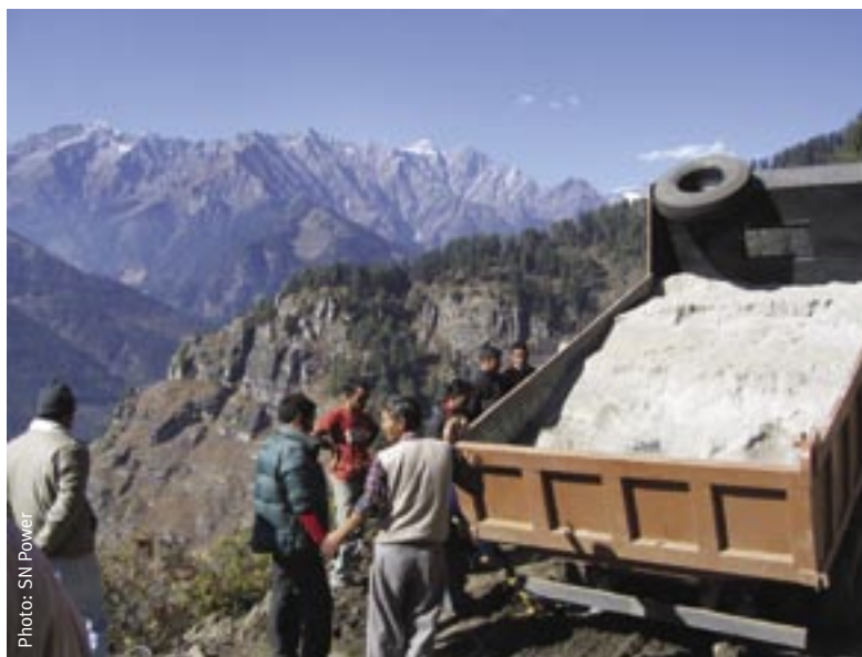
Building a road to Allain Duhangan, the largest foreign investment in Indian hydropower.
