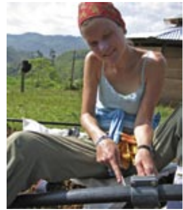
Marit Mastad tightens up a pipe in a water project in Chiapas, Mexico
