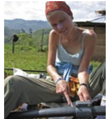
FK participant Marit Mastad tightens up a pipe in a water project in Chiapas, Mexico
