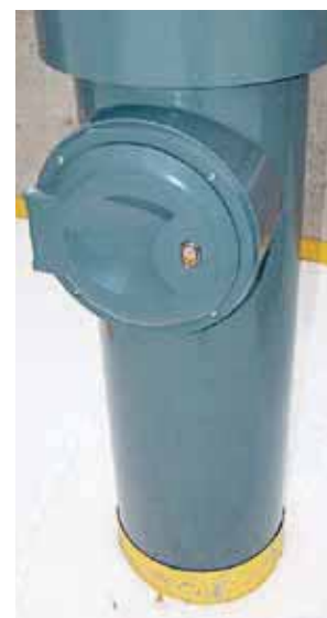
The vacuum-based waste system is discrete and practically located between two of the buildings
