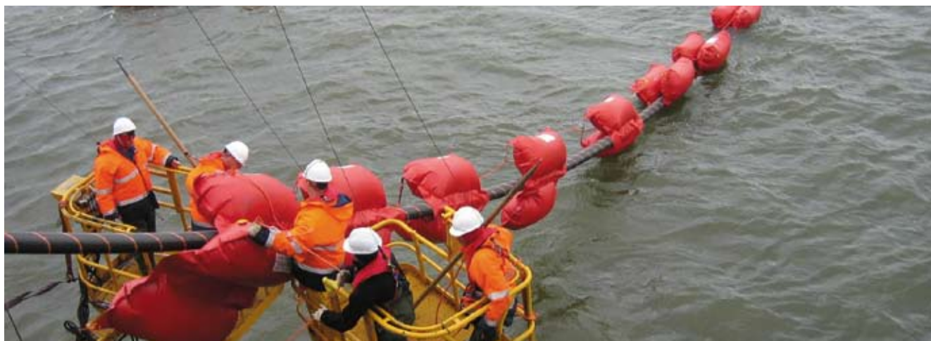
NorNed consists of a total of eight sections of cable. The first section was laid outside Eemshaven in the northern Netherlands in spring 2006. The entire cable had been laid and jointed by autumn 2007.
