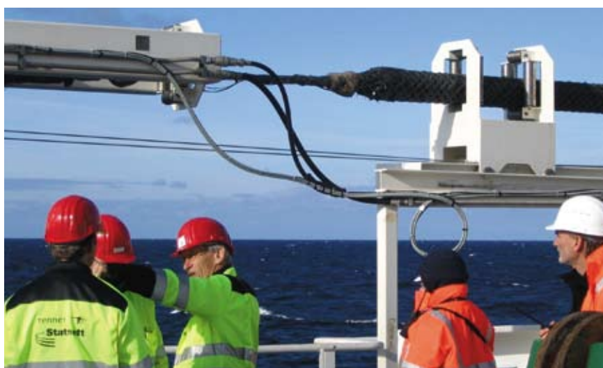
Between 2006 and 2007, cable was laid on the entire 580 km stretch between Norway and The Netherlands. The NorNed cable is almost twice as long as the world's second-longest submarine power cable between Tasmania and Australia.
