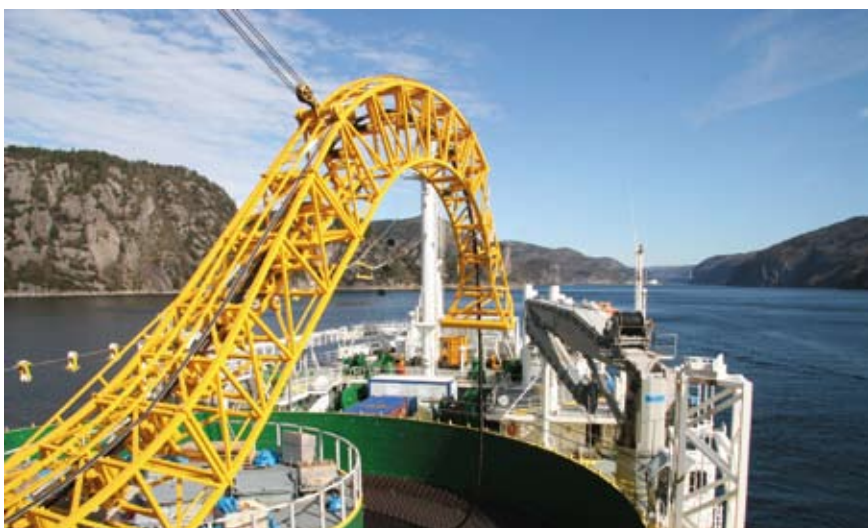
The entire section was laid and jointed in autumn 2007. On the way into the Fedafjord, the cable passed its deepest point at 410 meters.
