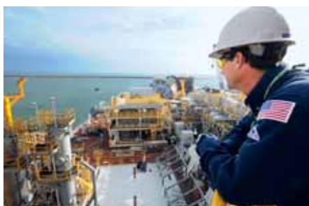
US Gulf of Mexico. At the yard in Corpus Christie, work is underway to complete the Tahiti platform.
