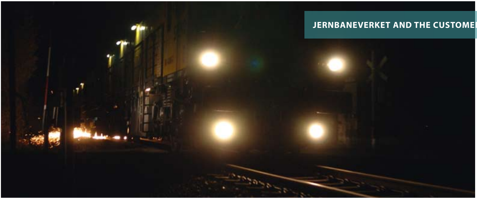
Overnight work: Rail grinding often takes place at night. The grinding train is 100 metres long and weighs 300 tonnes.
