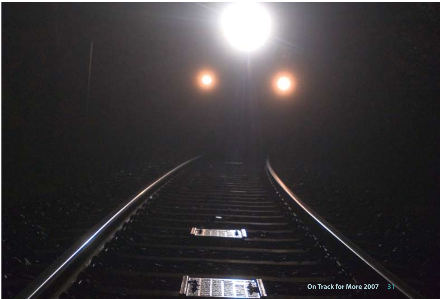
ATC beacons: Mounted on sleepers, these communicate with the train's ATC system and are used in signalling systems to monitor train speeds.
