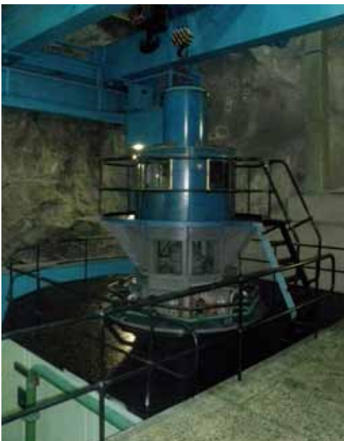
Turbine with generator at Hale Hydropower Plant
