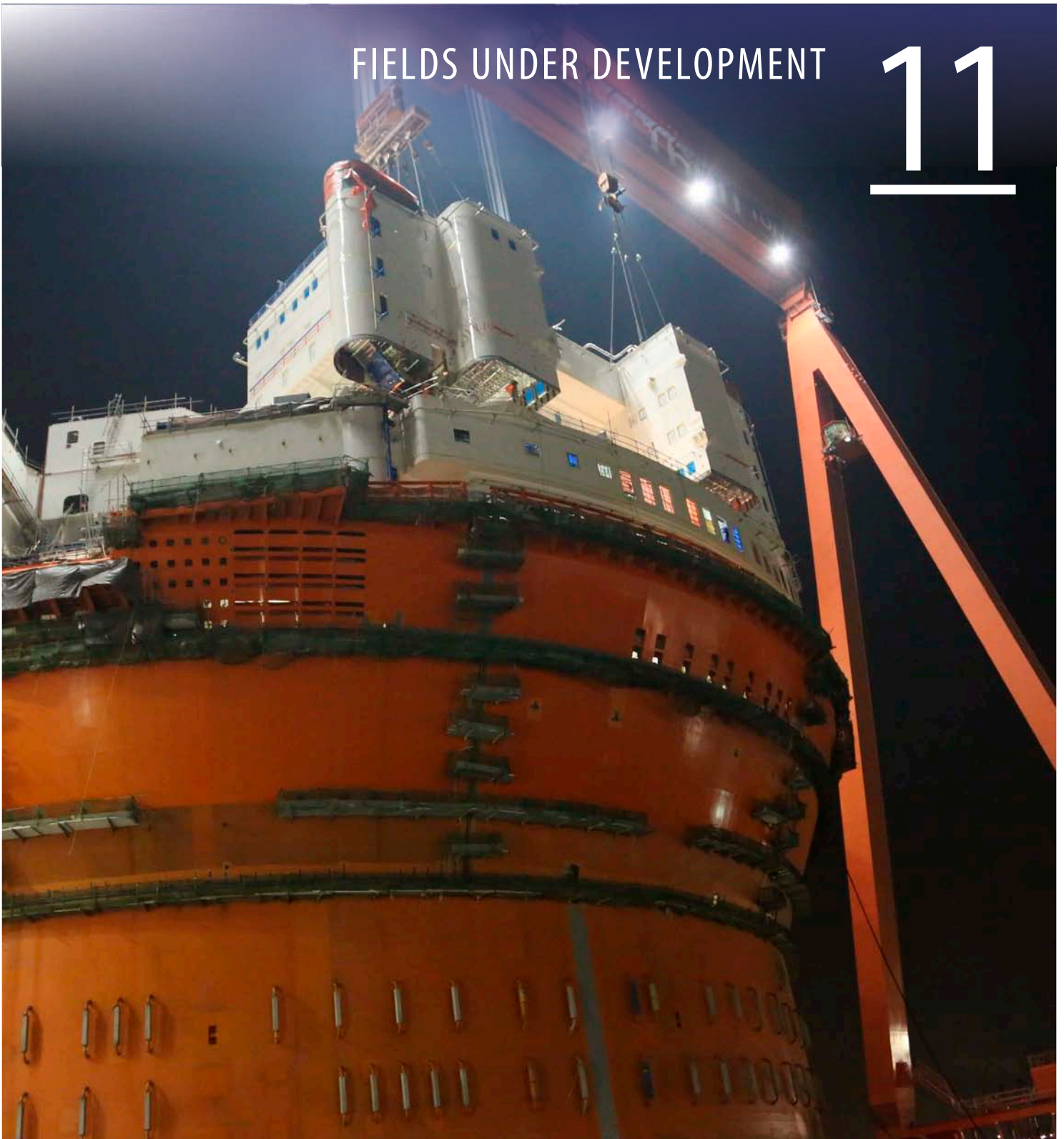
The living quarter is lifted into place on the Goliat facility, which is currently under construction at the Hyundai yard in South Korea. (Photo: Eni Norge, News on request)
