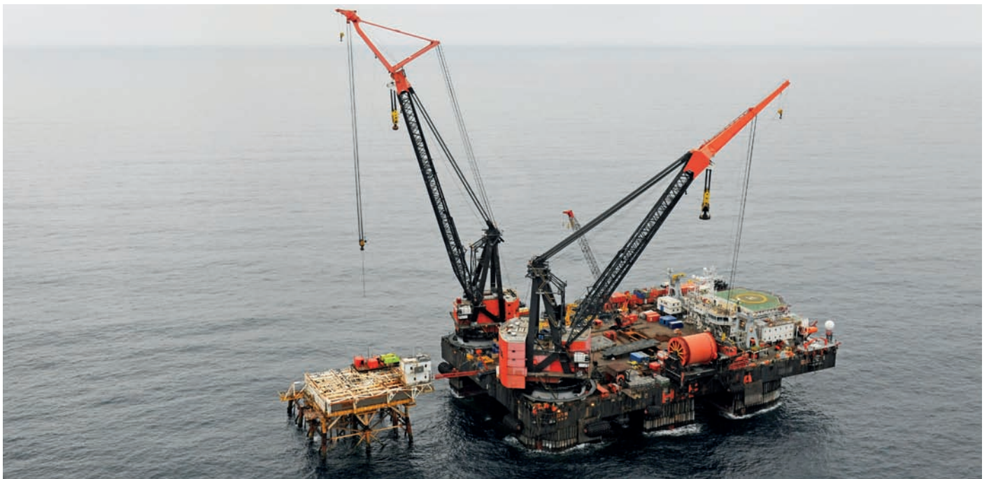
Figure 6.7 The Balder heavy lift vessel prepares removal of the Edda topside frame (Photo: Kjetil Alsvik, ConocoPhillips)
