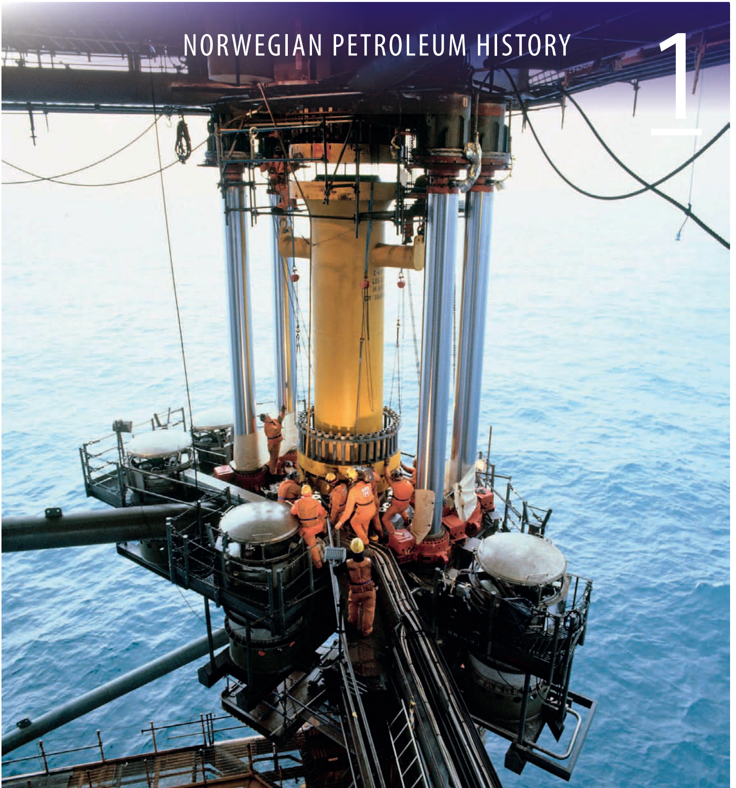
From the jacking up of the Ekofisk platforms in 1987. Here a piece is being put in place to extend one of the legs on the Ekofisk 2/4 hotel facility. (Photo: Husmo, ConocoPhillips/Norwegian Petroleum Museum)
