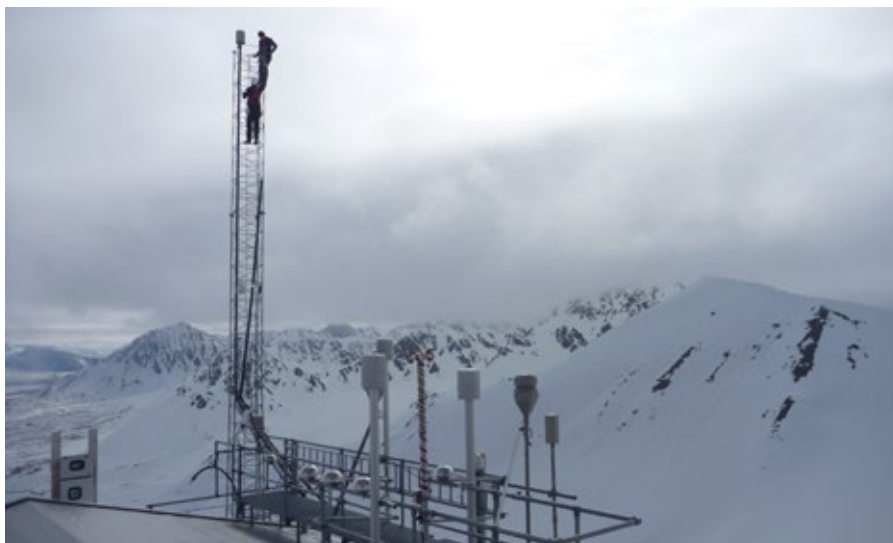
Ove Hermansen and Are Bäcklund from NILU installs air inlet on the mast at NILU's Observatory on Zeppelin Mountain, Ny-Ålesund. Photo: Sanja Forsström, Norwegian Polar Institute
