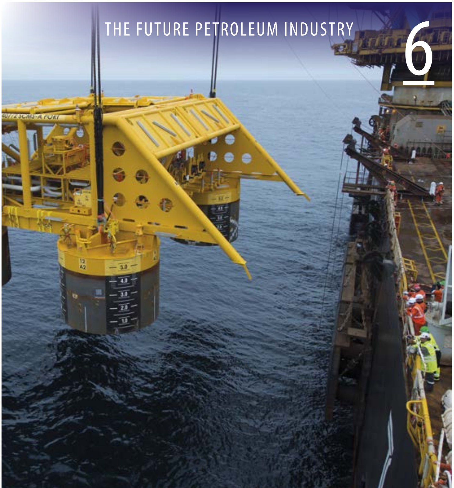
Installation of subsea compression equipment on the Åsgard field in the Norwegian Sea. This is innovative technology that will contribute to a substantial increase in gas and condensate production from the field (Photo: Øyvind Hagen, Statoil)
