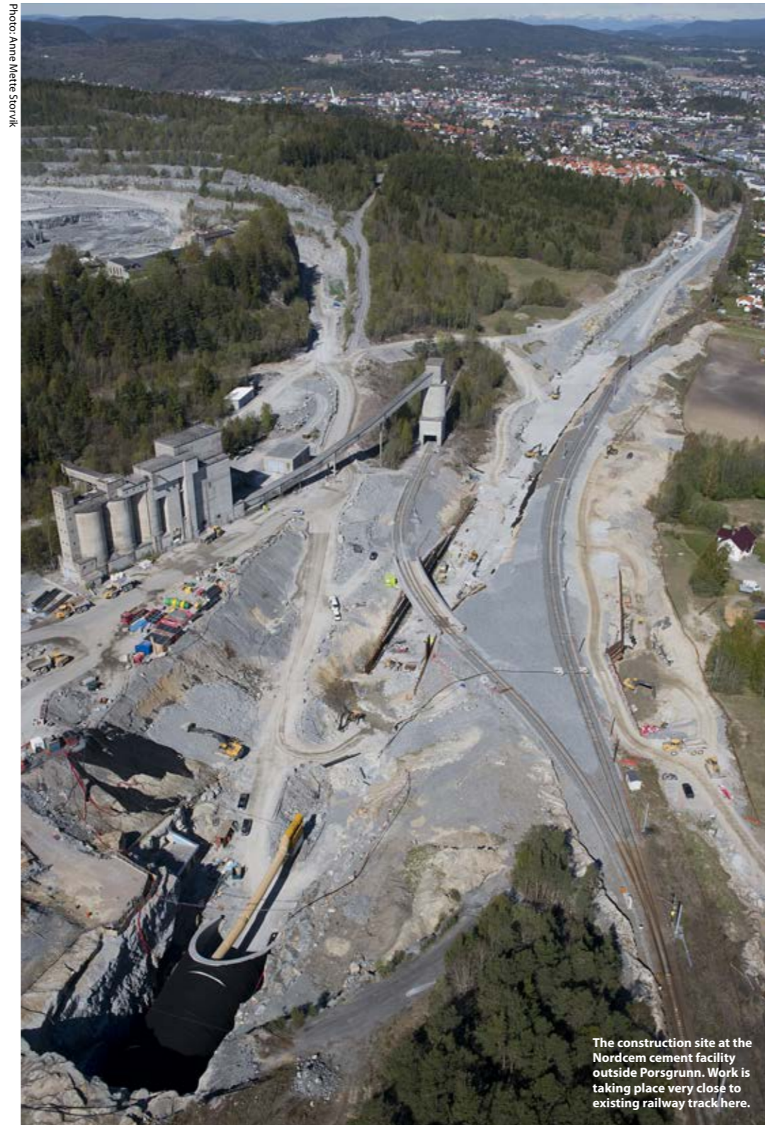
Seven tunnels and ten bridges have to be put in place in order to build a double track across the valleys between Farriseidet – pictured – and Porsgrunn.
