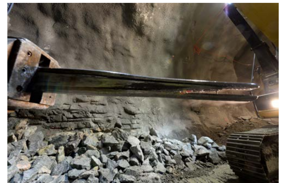
Italian tunnel specialists are using "Drill & split" – or mechanical rock breaking – to create an access tunnel for the Follo Line in Ekebergåsen from Sorenga. When a boring rig has bored up to 500 holes, what is known as a Superwedge splitter equipped with a wedge of around one metre will be used. This method does not cause vibration, but it is time-consuming; with progress of just one metre a day as compared to 10-15 metres in the case of standard blasting.
