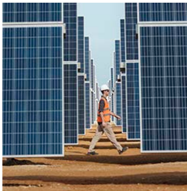
Apodi solar plant, Brazil.
