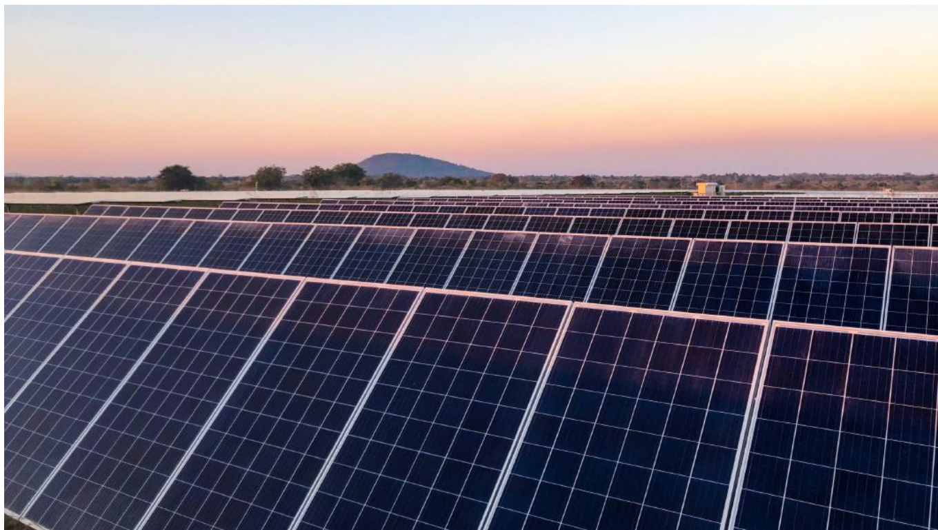
Central Solar de Mocuba, Mozambique
