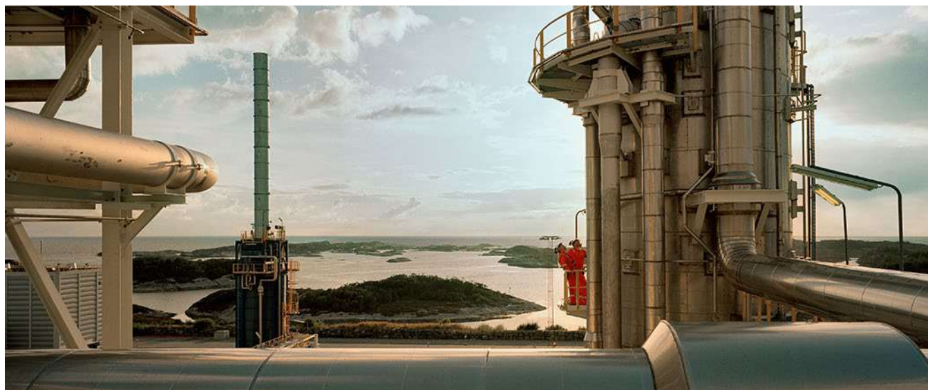
Kollsnes gas processing plant at Øygarden, Norway.
