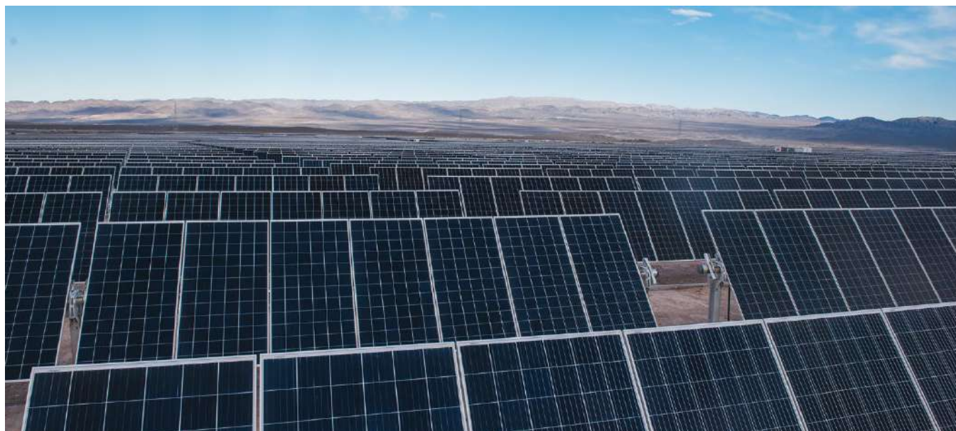
Guanizul 2A solar plant in San Juan, Argentina.
