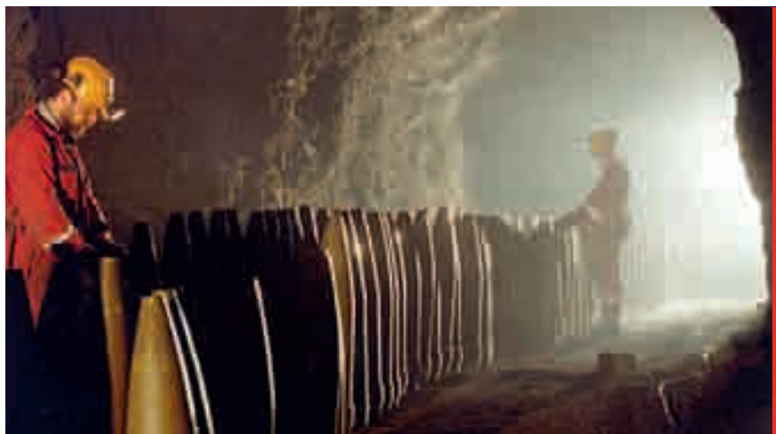
Preparing for underground detonations at Nammo NAD AS, Løkken Verk in Norway. Source: Nammo AS.
