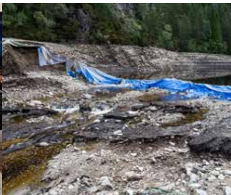
Dambrot Munkebotn i Bergen Foto: Rune Engesæter, NVE
